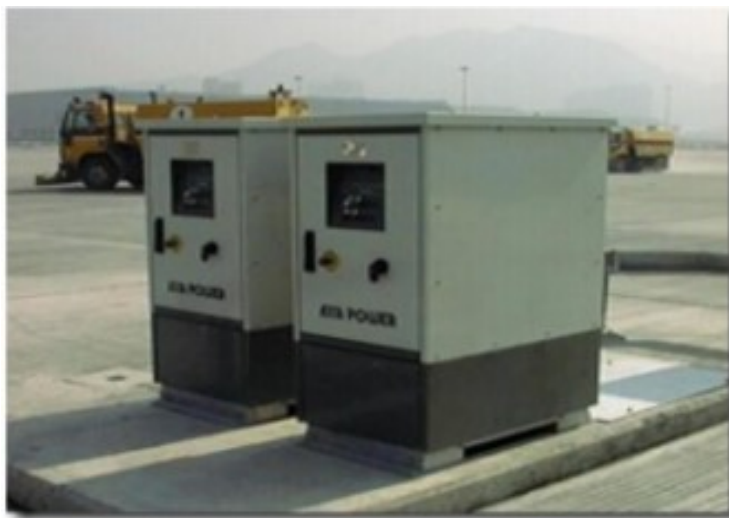
Two 90 kVA point of use frequency converters
