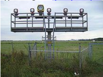
The approach lighting system of Bremen Airport
