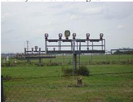
Approach lighting systems
