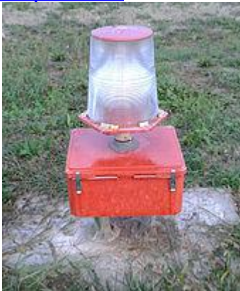
Runway end identifier lights
